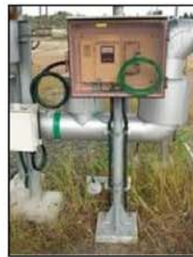
CO 2 detector (No leak)
