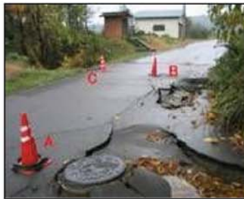
Access road was damaged.
